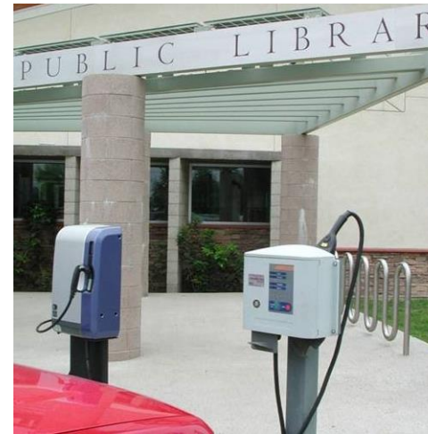
Electric vehicle charging stations at a Public Library
